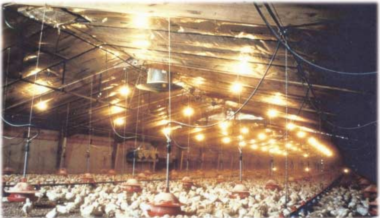
Radiant heat barrier - Chicken Farm, Philippines
